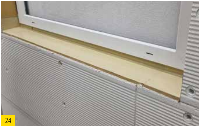
The ready glued and adapted sealing edge is now sealed at the butt joints and the render stop bead is fitted.
