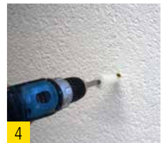
4 Flush insertion of the spiral anchor by means of a TORX T40 into the rendered wood fiber insulation board.
