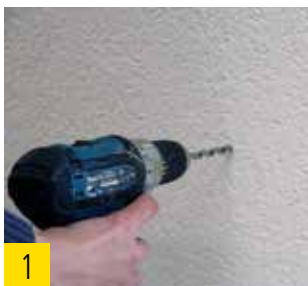
1 Pre-drilling of the rendered wood fiber insulation board by means of an 8 mm wood drill.
