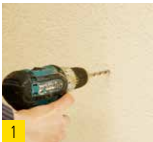
1 Pre-drilling of the unrendered wood fiber insulation board by means of an 8 mm wood drill.
