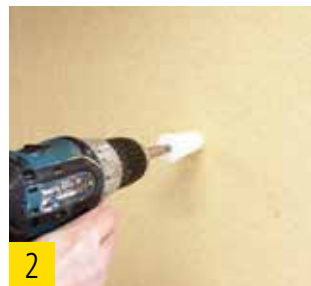
2 Insertion of the spiral anchor by means of a TORX T40 into the unrendered wood fiber insulation board.
