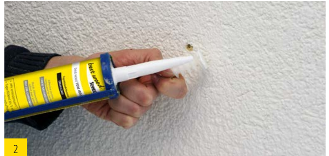
2 Application of best wood FDM WALL gap adhesive sealing compound for sealing purpose.
