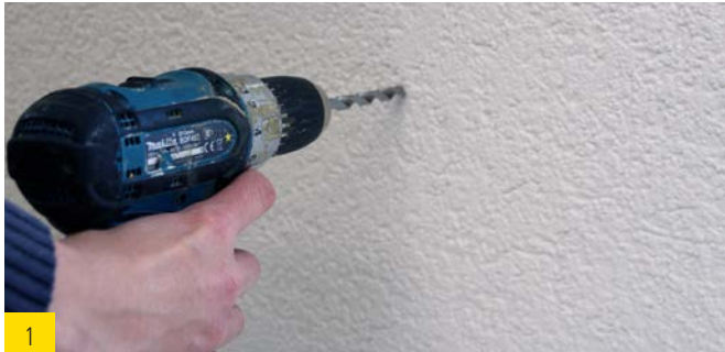
1 Pre-drilling of the rendered wood fiber insulation board by means of an 8 mm wood drill.
