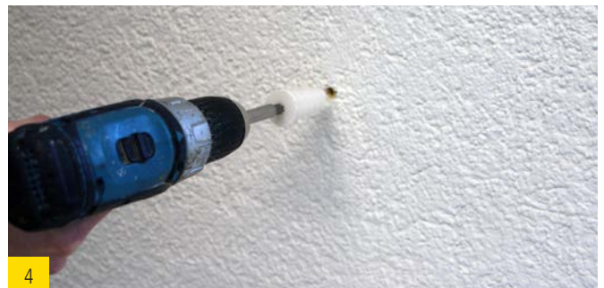
4 Flush insertion of the spiral anchor by means of a TORX T40 into the rendered wood fiber insulation board.
